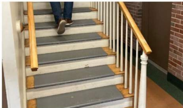
Inaccessible stairs lack code compliance.
