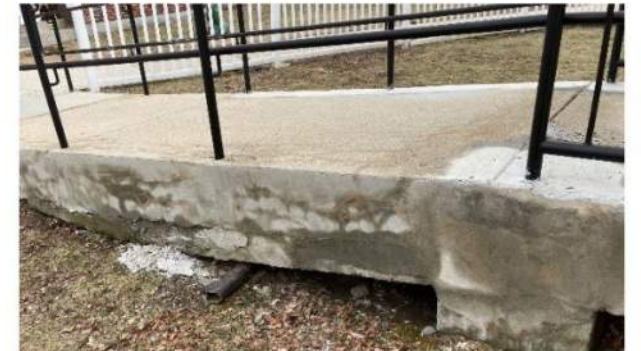
Damaged ramp with repeated failing repairs.
