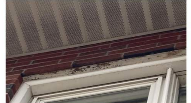
Rusted lintels and displaced bricks.
