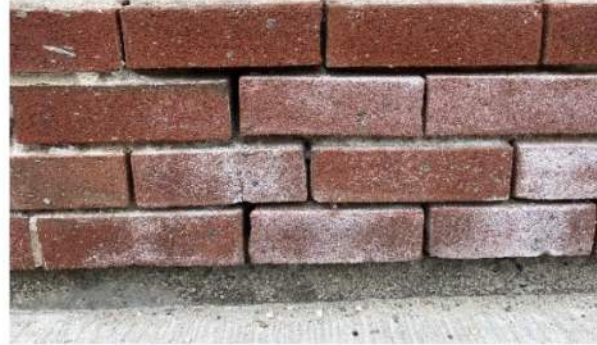
Degraded mortar and brick misalignment.
