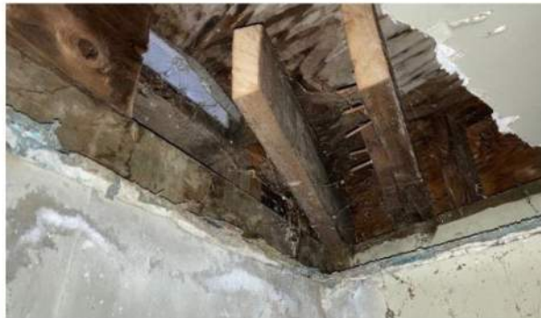
Floor framing rot and water damage.
